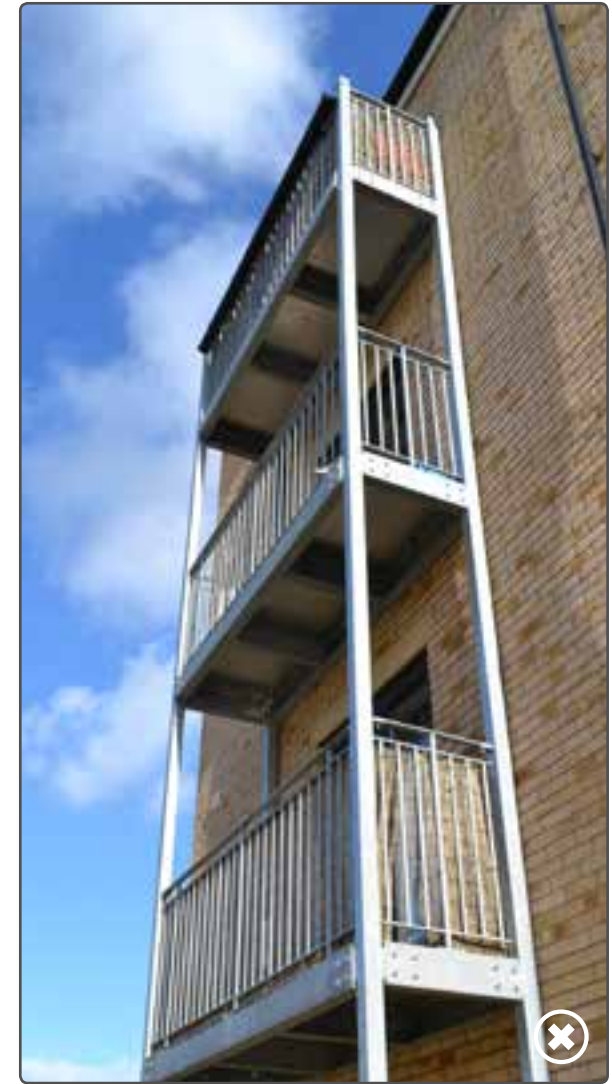
Poor external balcony design
