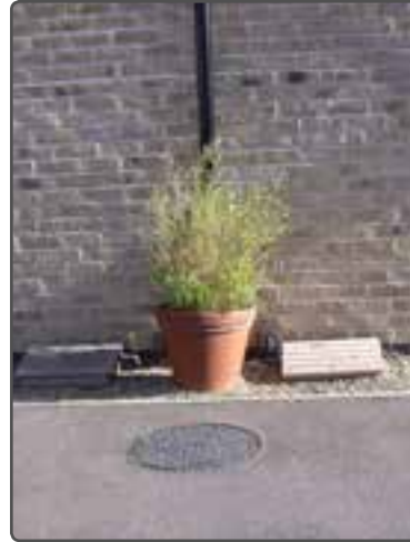
Semi concealed gas meter
